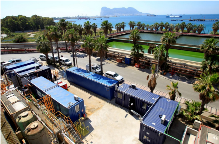
Figure 1. The MSAR manufacturing unit (in a 40 ft container; bottom left), and associated modules at Cespa's Gibraltar San Roque Refinery.
